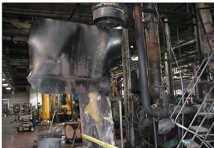
Air System Fire Induced Rupture
